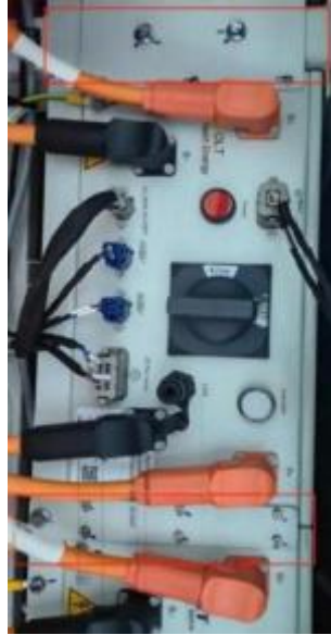
picture 9-20 High-voltage box fixed position
